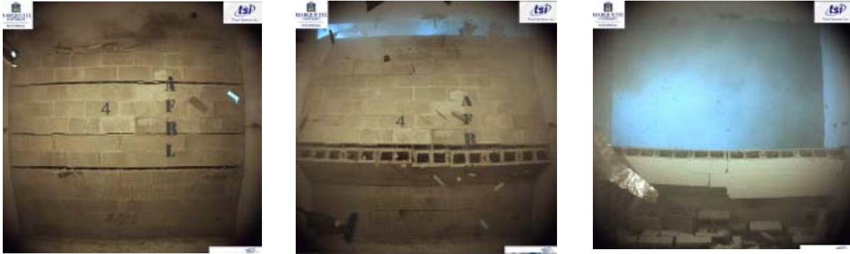
Unprotected walls can collapse and send dangerous debris into building.
